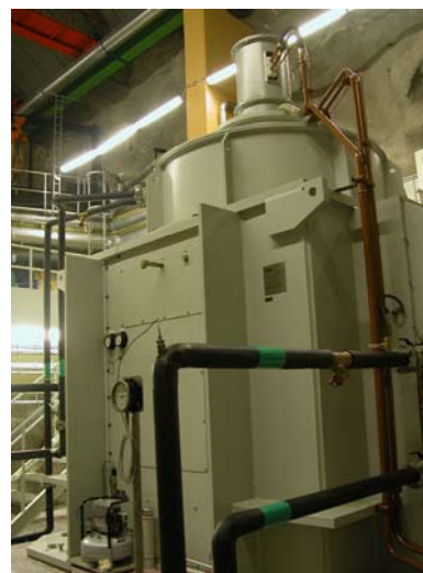
Fig. 2 Part of the generator
