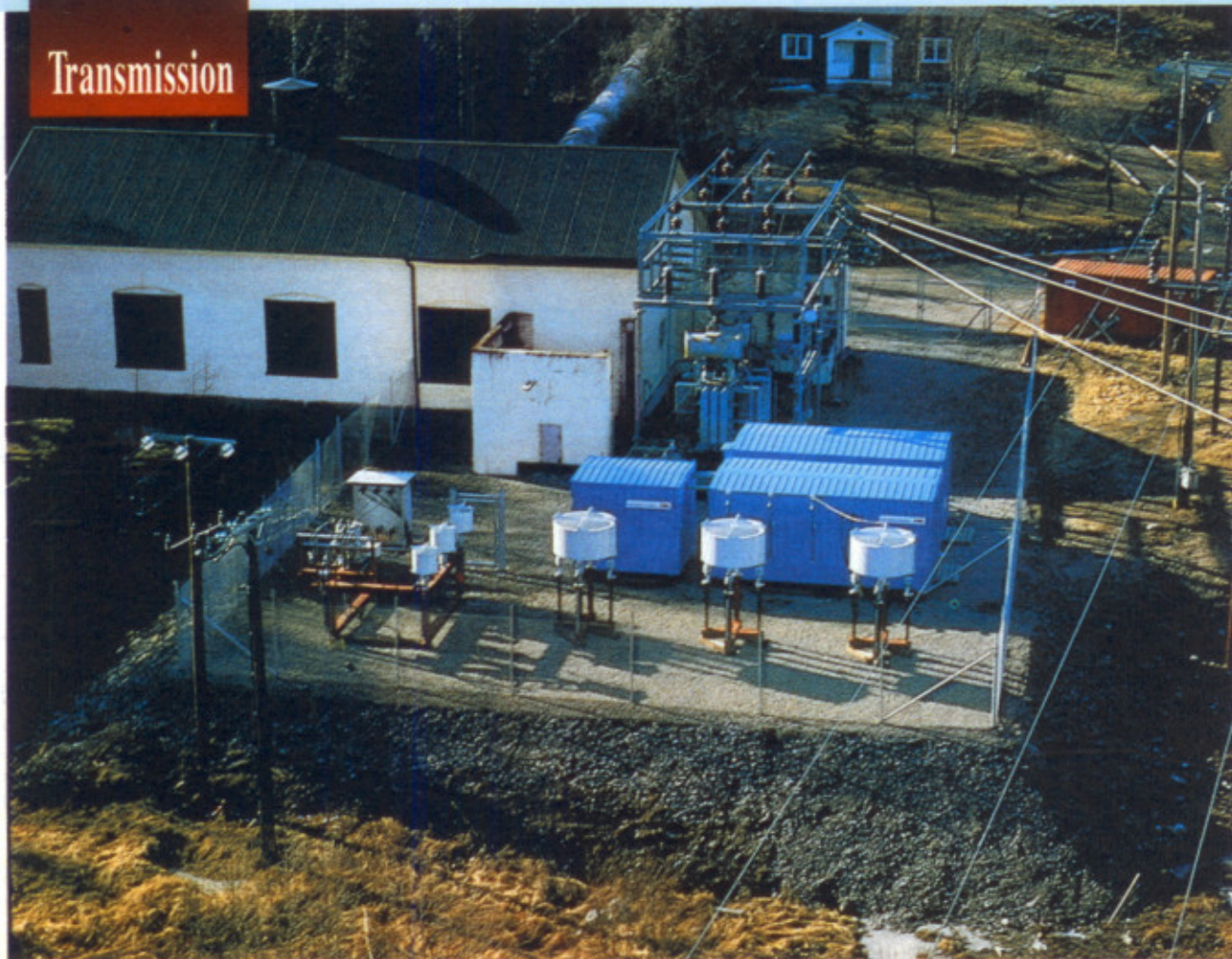
Fig. 1. The Hellsjön converter station.
